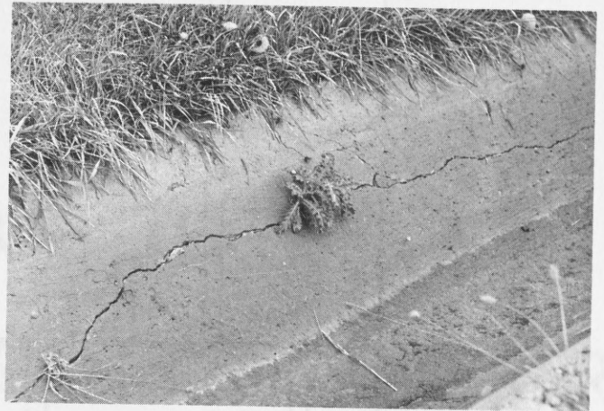
One of the longitudinal cracks that developed along the slip-formed concrete ditch lining.
